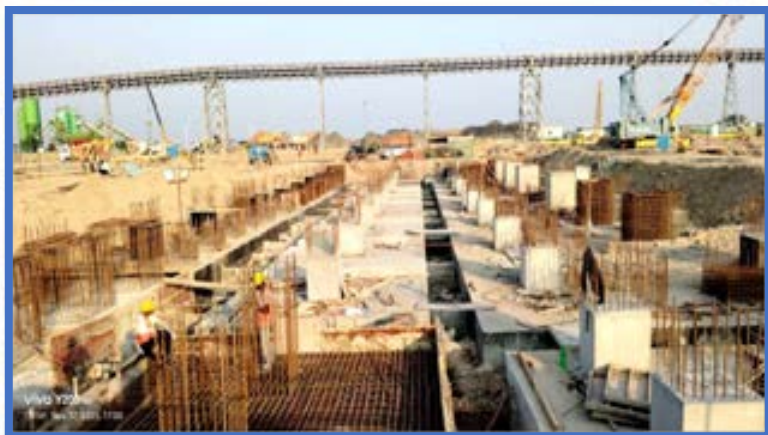
Chlor - Alkali Plant - HCl Desorption Train #2
