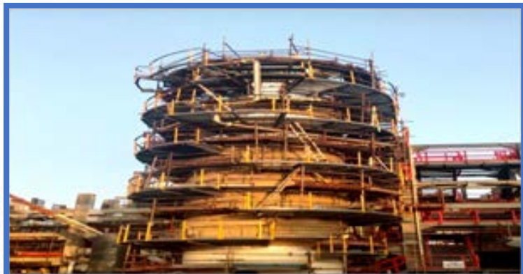
PVC Plant – Stripping Column
