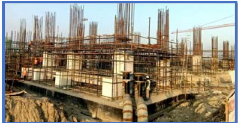
Chlor Alkali Plant - Rectifier Substation
