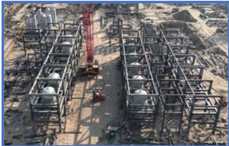
VCM Plant Train - 2
