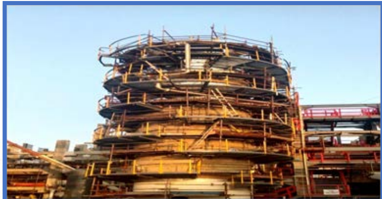
PVC Plant – Stripping Column
