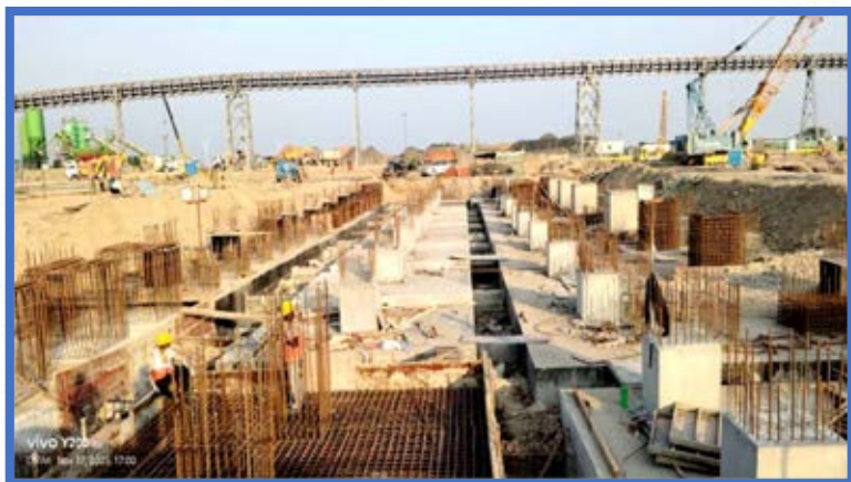
Chlor – Alkali Plant – HCl Desorption Train #2
