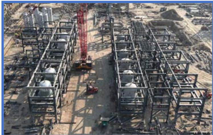
VCM Plant Train - 2
