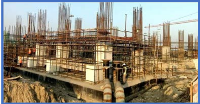
Chlor Alkali Plant - Rectifier Substation
