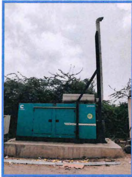
D.G. Sets having adequate stake height and Acoustic system covered on it.
