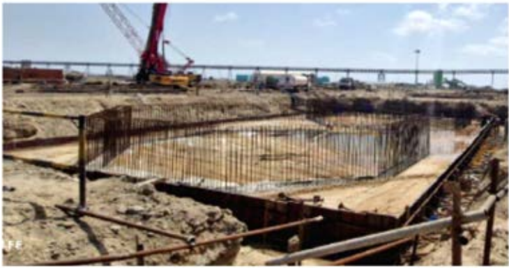
Chlor-Alkali Plant - Primary Brine Tank
