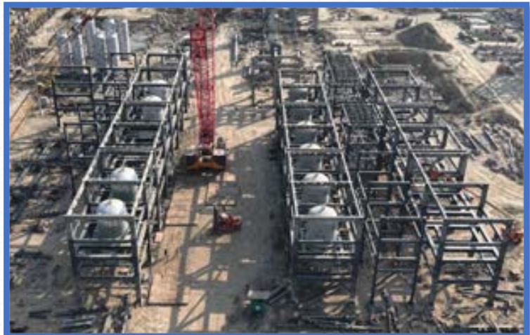
VCM Plant Train - 2
