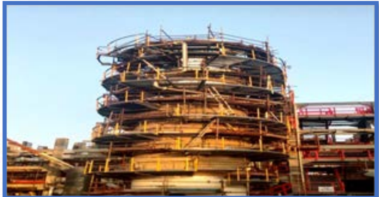
PVC Plant – Stripping Column
