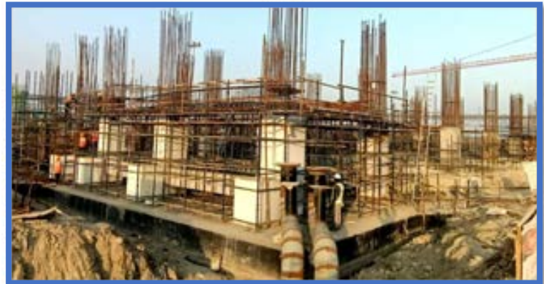
Chlor Alkali Plant - Rectifier Substation
