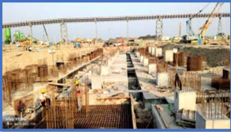
Chlor - Alkali Plant - HCl Desorption Train #2
