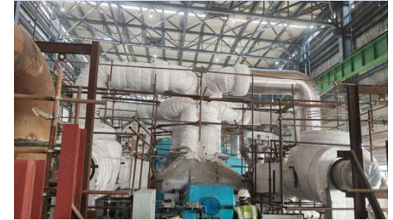
Unit #3- Induced Draft Cooling Tower
