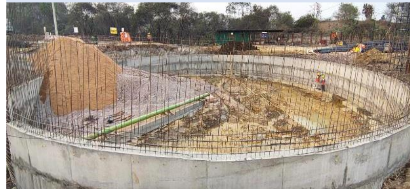
High-Rate Solid Contact Clarifier
