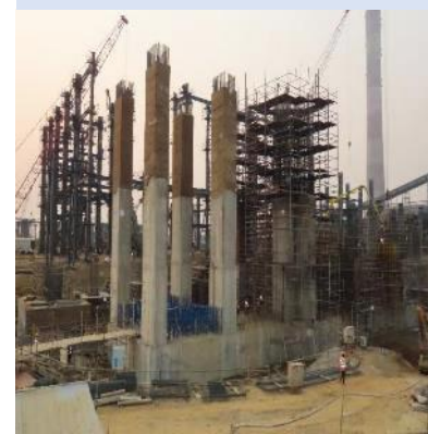
Unit #3 - Turbine Generator Deck
