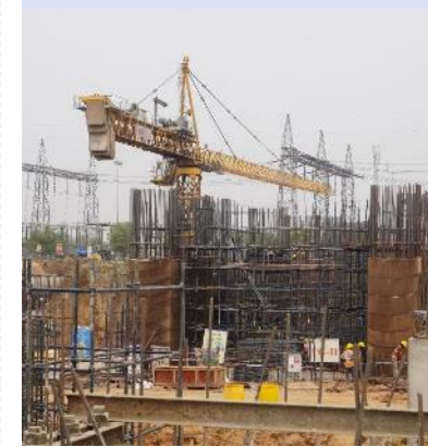
Unit #3 - Turbine Generator Deck
