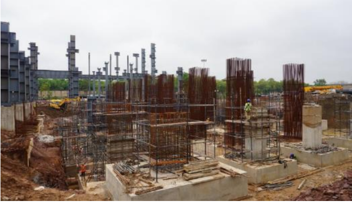
Unit #3 - Turbine Generator Deck
